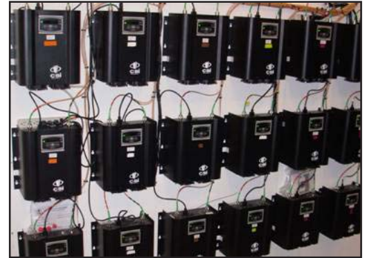
Bi-directional amplifiers (BDA) receives signal via fiber from cellular carrier base stations, which are then sent to the MobileAccess system on nearby racks and redistributed via the distributed antenna system installed in the stadium
