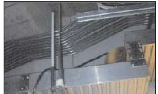
Twenty 450 MHz omnidirectional antennas are positioned around the stadium to enhance first responder communications. This one located under the stands
